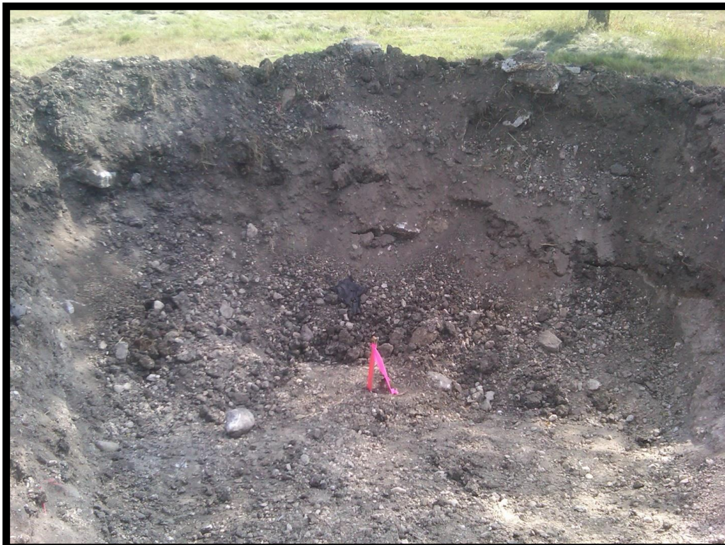
Figure 5. Picture of the abandoned well #1 after being excavated about 4 feet. The well is next to the stake with the pink flag.
