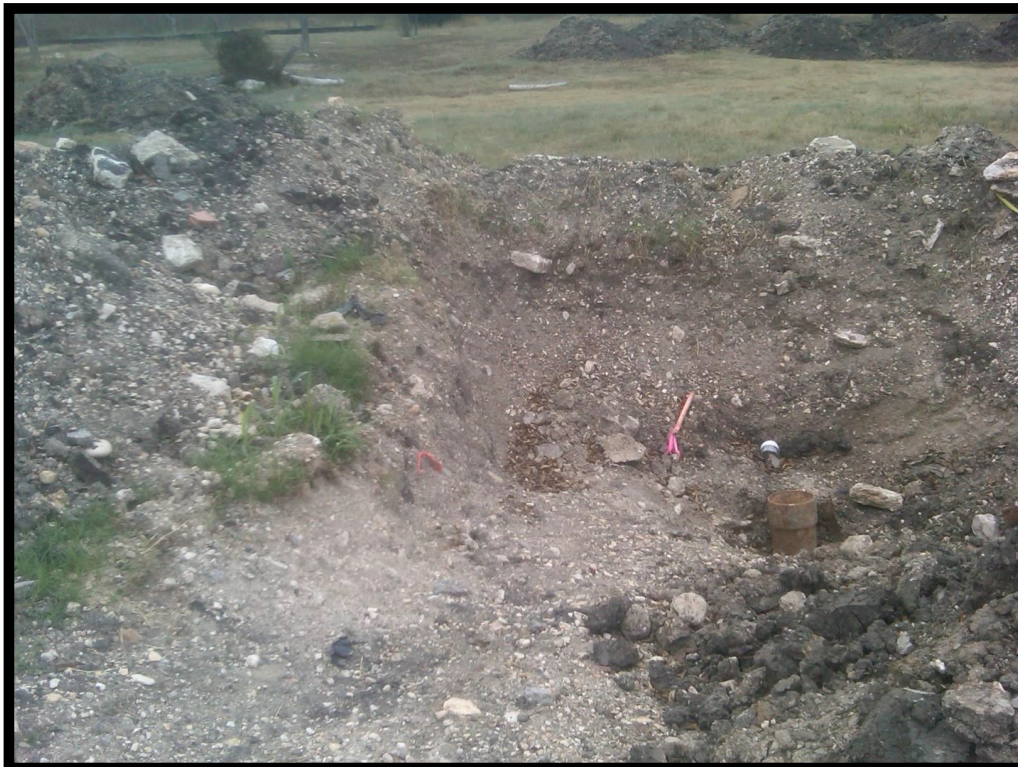
Figure 7. Picture of the abandoned well #2 after being excavated and exposed. It is located next to the stake with the pink flag.
